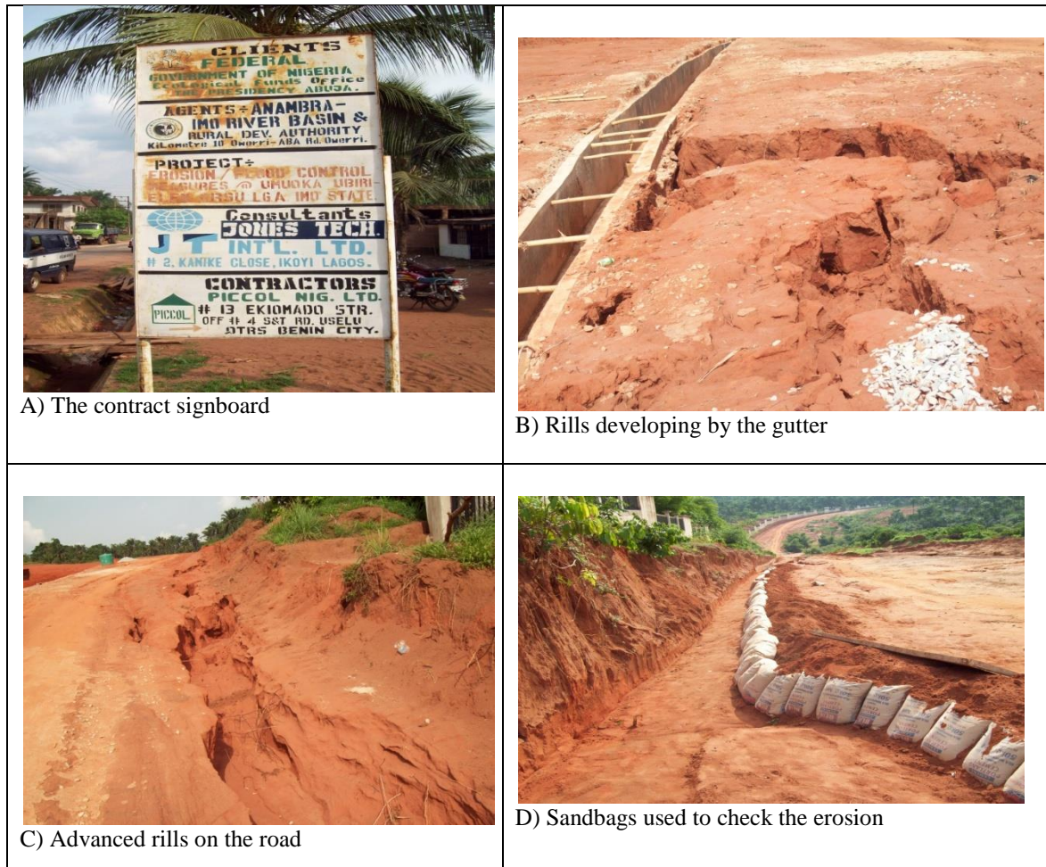
Figure 3: Umuoka Ubiri Elem erosion site
